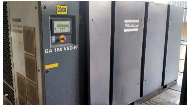
4765 - COMPRESSOR - GA 160 VSD FF ATLAS COPCO
